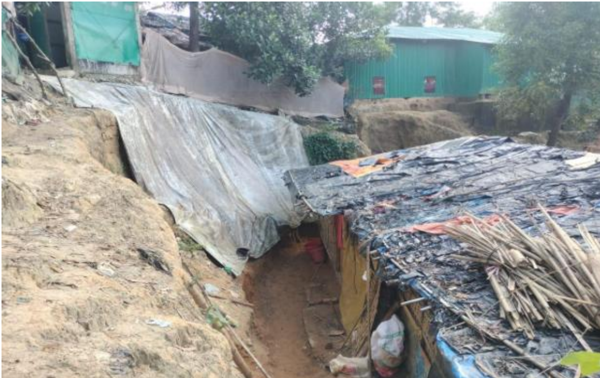
Before the intervention: An unstable slope in Camp 13 showing severe soil erosion and floodwater flowing directly toward nearby shelters, posing serious risks to families and children during the monsoon season
