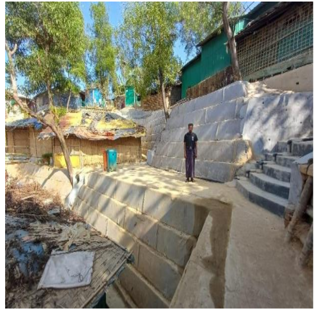
Mr. Samsu stands confidently beside the stabilized slope beside his home, reflecting the renewed sense of safety and dignity restored through the intervention.
