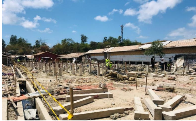
Construction of Composite Bamboo Shelters (CBS) on stilts in Block H, Camp 26
