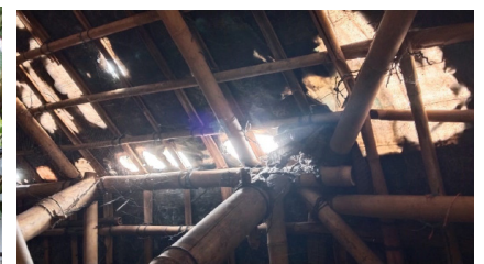
Image: Fully Damaged Shelter in Camp 18
