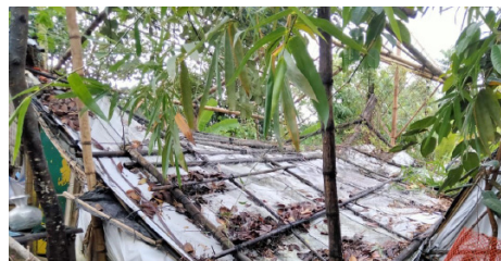
Image: Partially Damaged Shelter in Camp 19
