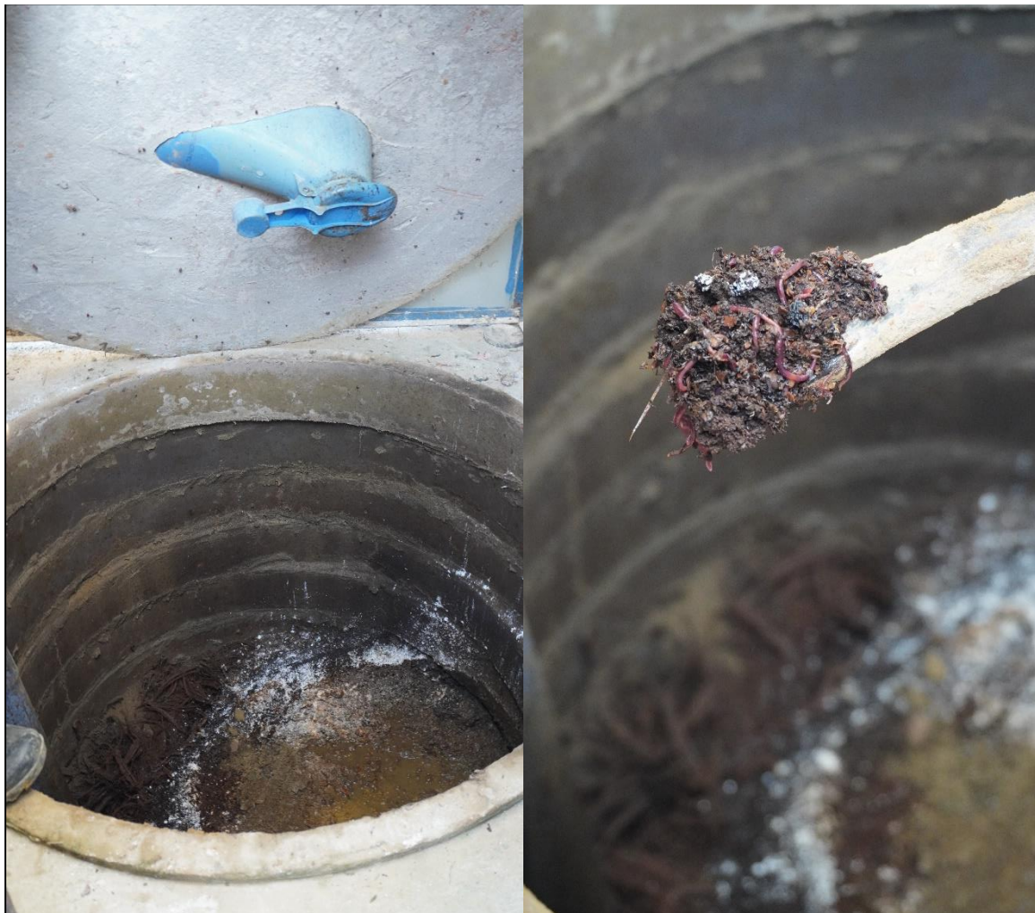
Photograph 2.13: Inside condition of digester of a Biofil toilet at Camp-27, Teknaf Nayapara Camp (ID: Teknaf-Camp 27(B)-SL4-ID-69) where Tiger worms were detected in the digester
