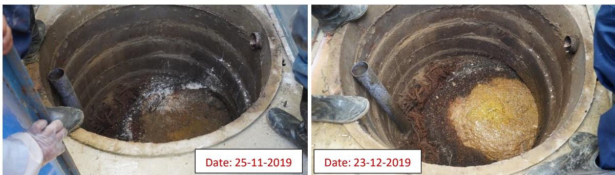
Photograph 2.7: Inside condition of digester of a Biofil toilet at Camp-27, Teknaf Nayapara Camp [ID: Teknaf-Camp 27(B)-SL4-ID-69]
