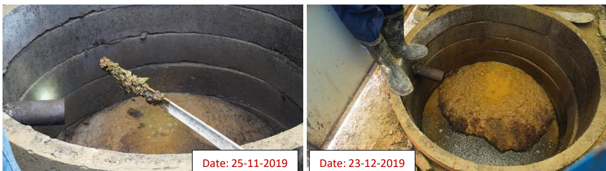
Photograph 2.8: Inside condition of digester of a Biofil toilet at Camp-27, Teknaf Nayapara Camp [ID: Teknaf-Camp 27(B)-SL2-ID-47]
