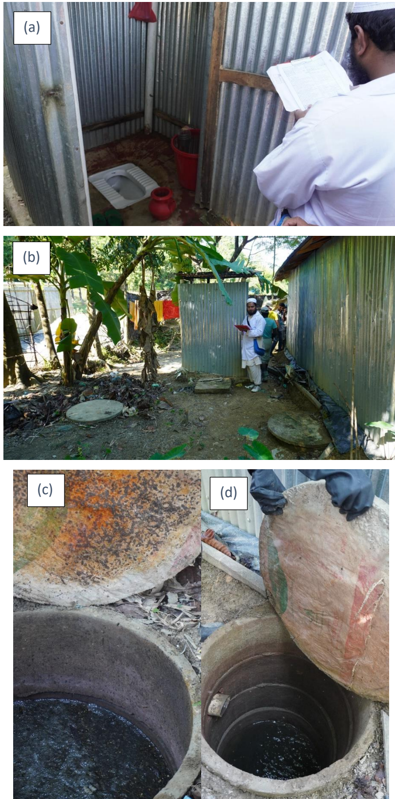
Photograph 2.5: BRAC constructed 2.5" dia alternative twin pit pour flush toilet at host community adjacent to Camp-22, Teknaf Whykong Camp (ID: Teknaf-Camp22 (Host)-SL6-HH-ID-1052) [(a): inside condition of alternative twin pit toilet, (b) backside view (c) used pit, & (d) pit not currently in rest]
