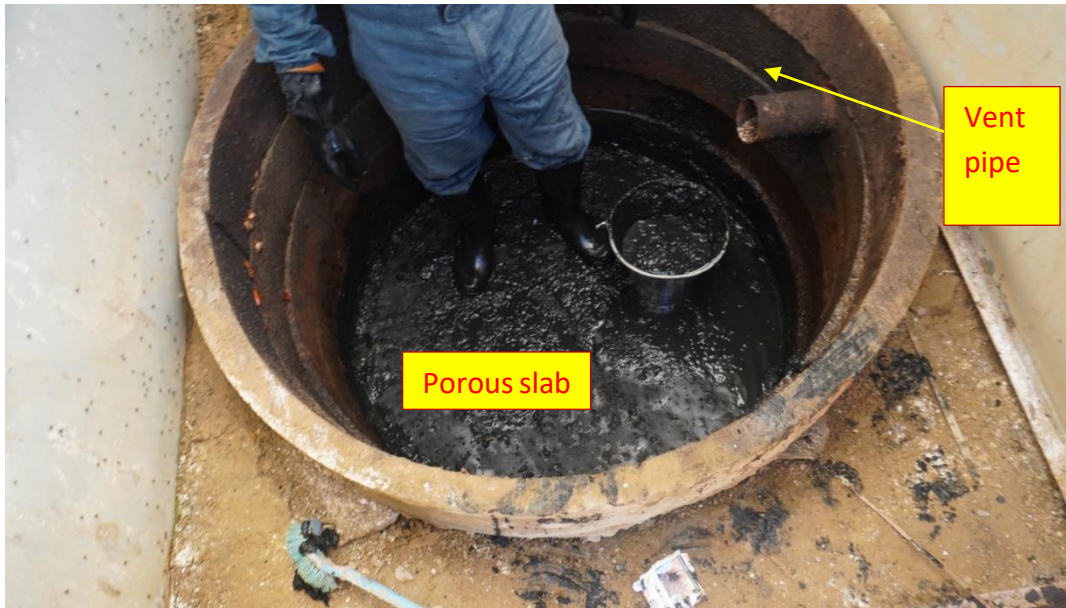
Figure 3.2: Positioning of vent pipe and porous slab for Type-1 Biofil toilet; photograph taken during desludging operation
