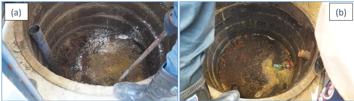
Figure 3.11: Good condition of digester for Type-1 [(a) ID: Teknaf-Camp27(B)-SL4-ID-69; (b) ID: Ukhia-Camp19(C-14)-SL1]
