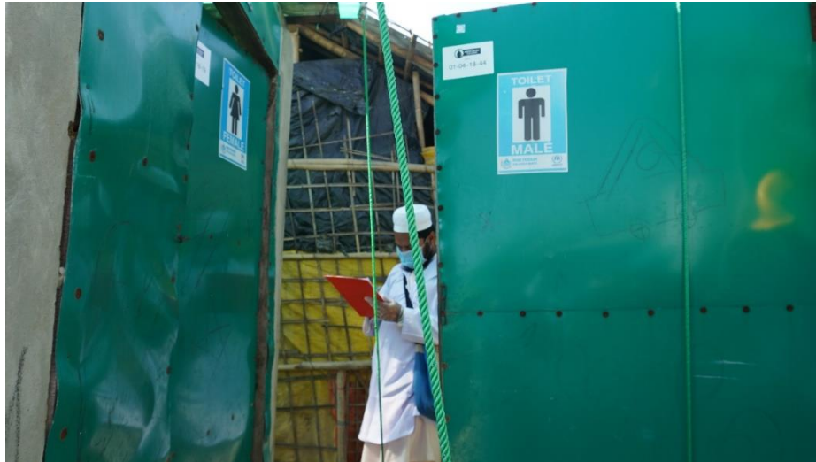
Photograph 2.2: NGO-Forum constructed 48” dia Twin pit pour flush latrine at Camp-26, Teknaf Nayapara Camp [ID: Teknaf-Camp26(A)-SL10 –ID-42]
