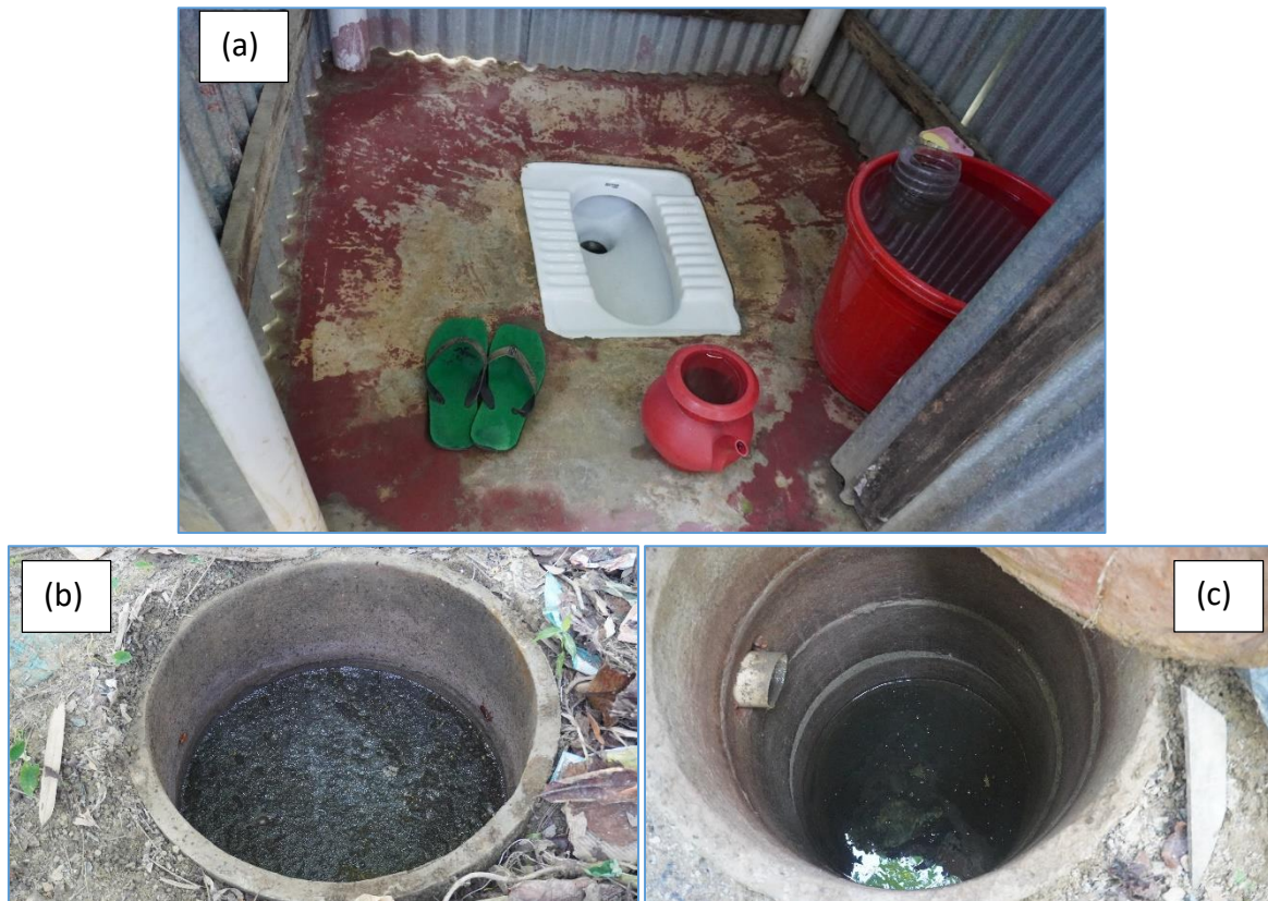
Figure 3.8: Inside view of alternative twin-pit latrines with 2.5 ft diameter concrete rings (a); [(b) operational pit, (c) pit in rest]
