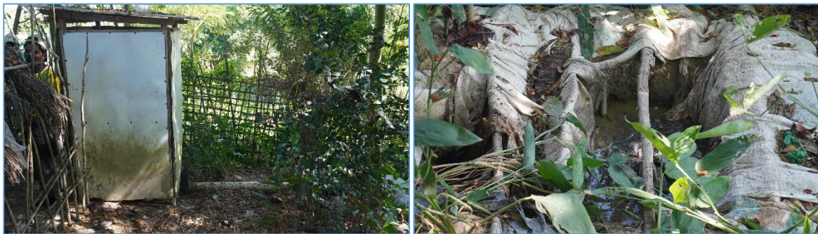
Figure 3.9: Biofil toilet in the host community of Camp-22, Teknaf [ID: Teknaf-Camp22 (Host)-SL1], failed to fulfil the criterion of presence of vent pipe
