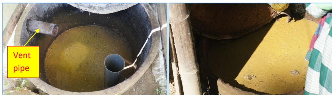
Figure 3.5: Positioning of vent pipe for Type-2 Biofil toilet (a) & Sludge in digester builds-up to clog the vent pipe (b)
