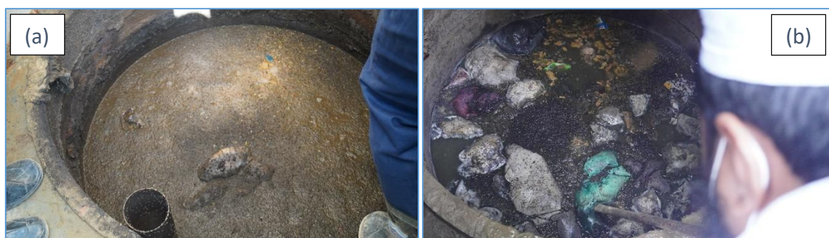
Figure 3.10: Accumulation of water on top of digester for Type-1 [(a) ID: Teknaf-Camp 26(A)-SL8-ID-Nil; (b) ID: Taknaf-Camp 27-SL7-ID-104]
