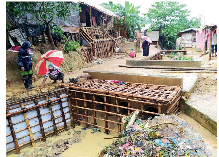
Bamboo waste trap installed to avoid the blockage of the pipe culvert
