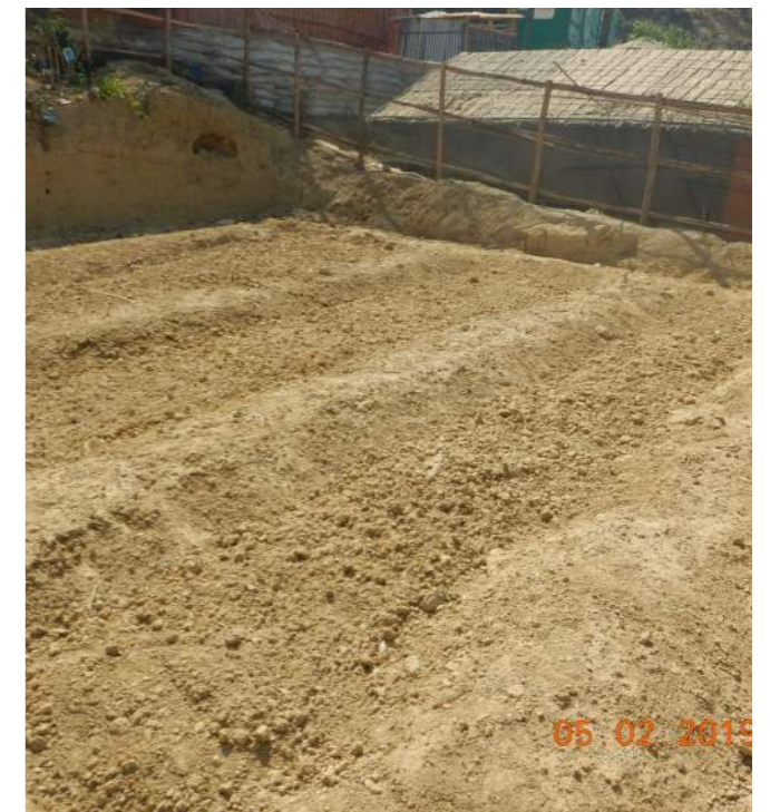
Image 42: Lime 5 - liquid infiltration trenches
