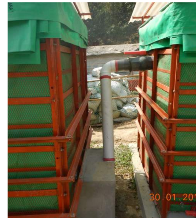
Image 3: Plant 2 (NGO 1) - Pipework between filters
