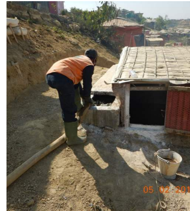
Image 39: Lime 5 - Inlet and Lime mixing point
