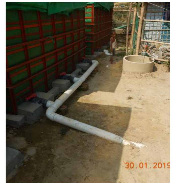
Image 4: Plant 2 (NGO 1) - Solids removal pipework
