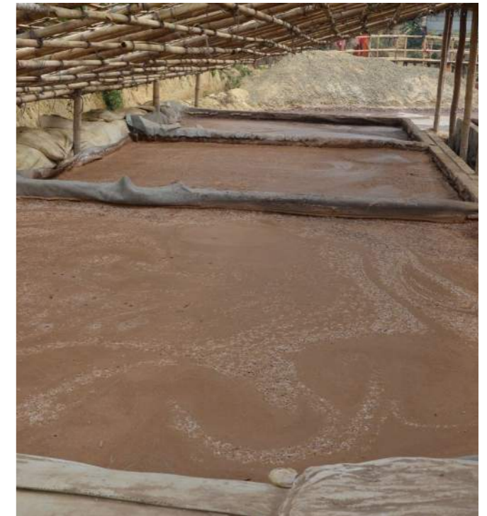
Image 25: Lime 1 - Dewatering bed
