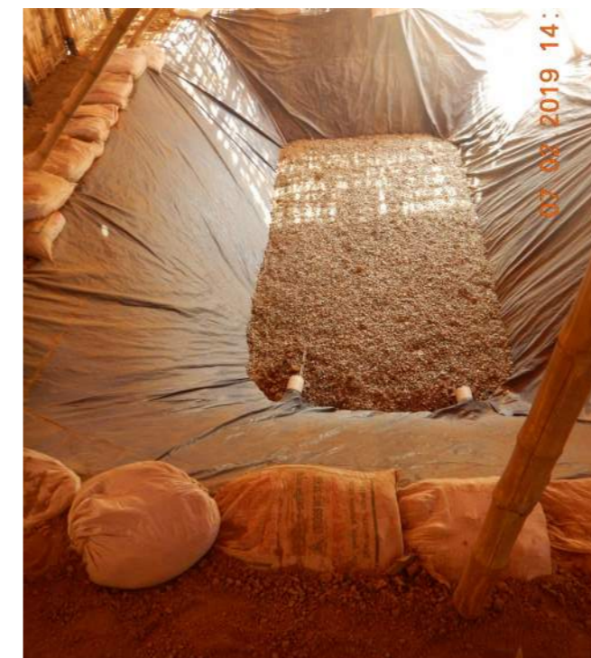
Image 34: Lime 3 - Gravel filter/dewatering bed
