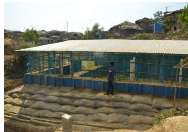
Image 13: Constructed Wetland external view
