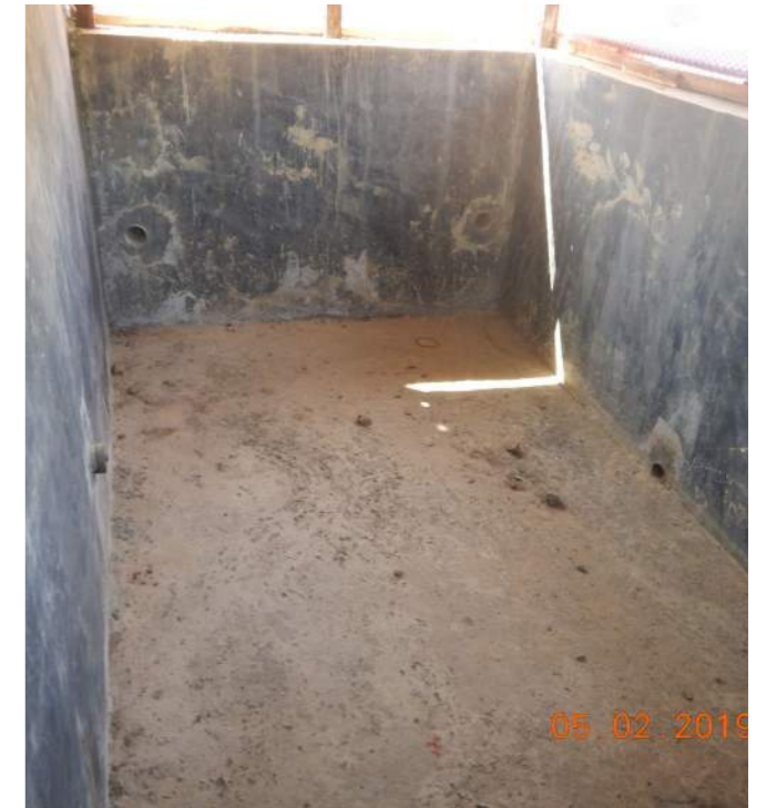
Image 40: Lime 5 - Lime holding tank ( 1 of 3)
