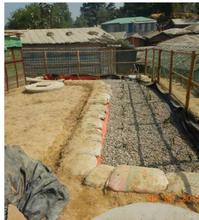
Image 2: Plant 1 (NGO 1) - Constructed Wetland liquid treatment
