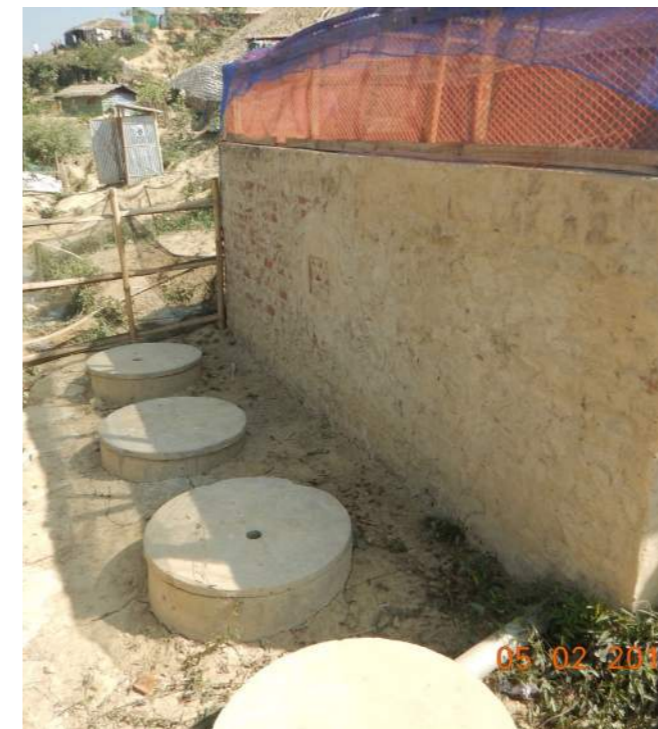
Image 41: Lime 5 - Solids storage pits
