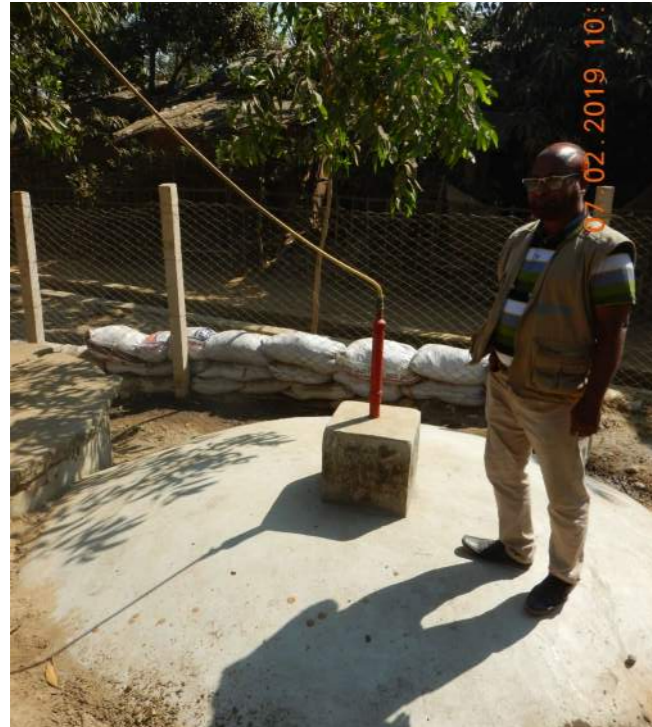
Image 17: 4m 3 concrete biogas digester
