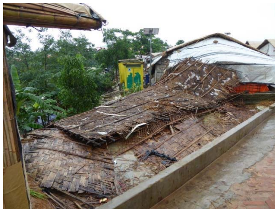
Photo 8.3.3: Collapsed shelter, camp 4, June 2021
