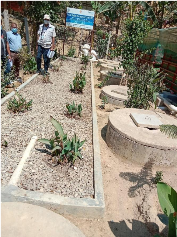
Planted filter and solids pits
