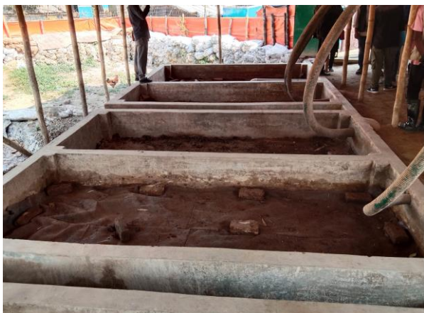
Drying and dewatering beds
