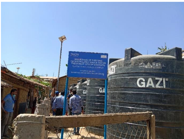
Biodigester and UFF tanks
