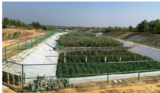
Planted drying bed
