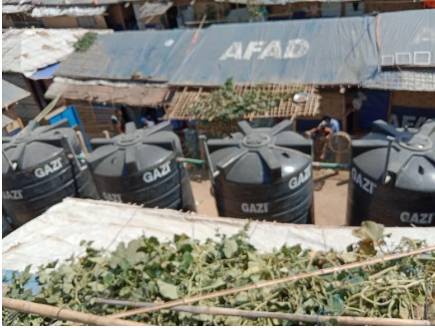
Biodigester and UFF tanks
