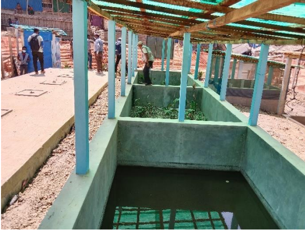
UFF and gravel filter
