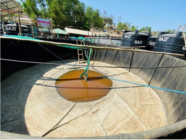
Final settlement tank
