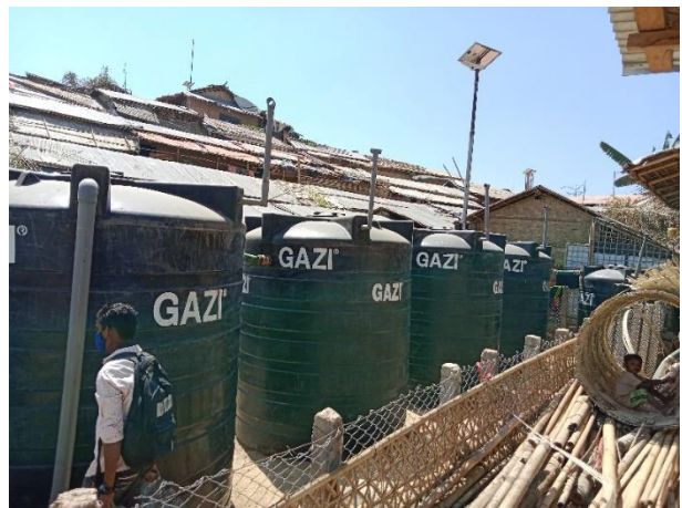
Biodigester and UFF tanks
