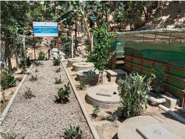
Planted filter and solids pits
