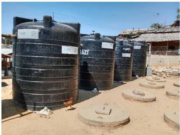
Biodigester and UFF tanks
